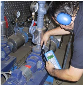
Figure 4 - Monitoring feed water pump
